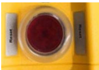
Fig. 8: Illuminated pushbutton fault
